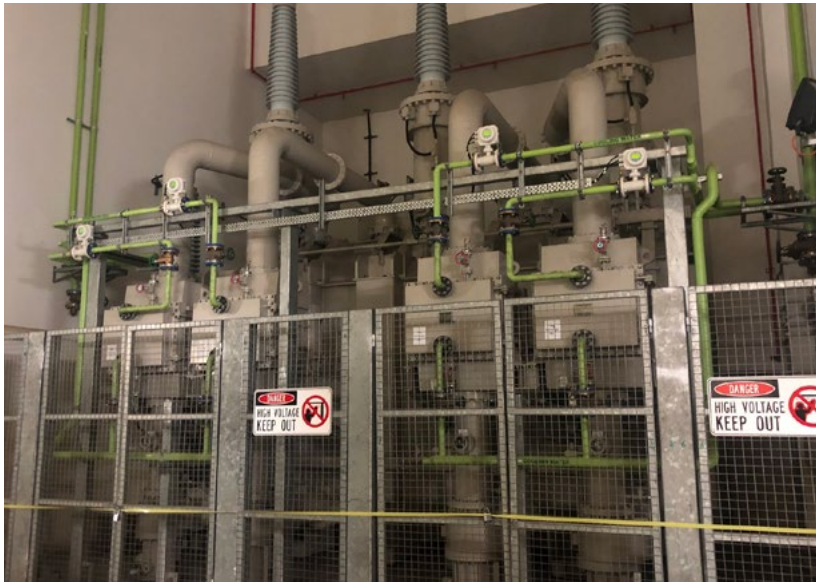
Ausgrid is implementing an SF 6 strategy to reduce use and losses of this gas.
