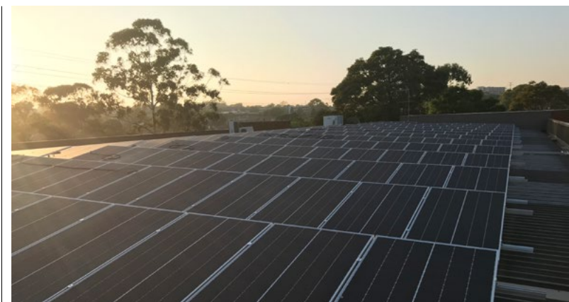
Ausgrid solar panels at Homebush.
