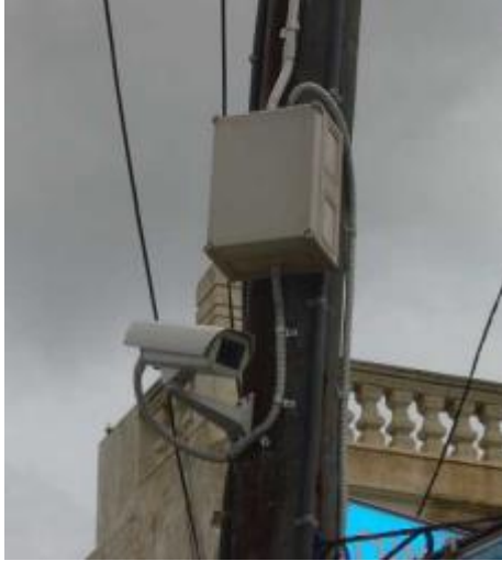
Figure 9: Typical CCT installation
