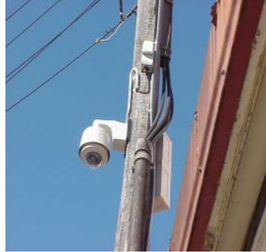
Figure 10: Typical wireless camera installation with mini panel antenna mounted above
