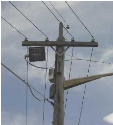
Figure 7: Single spot light mounted directly on LV cross arm
