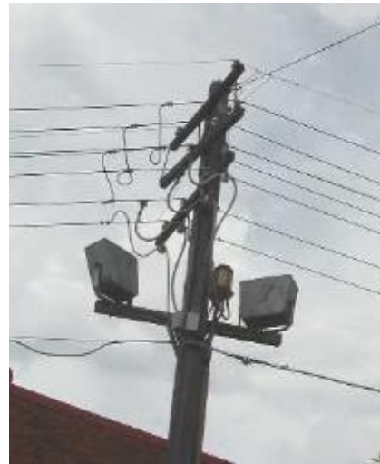
Figure 8: Pair of security flood lights mounted on a separate cross arm
