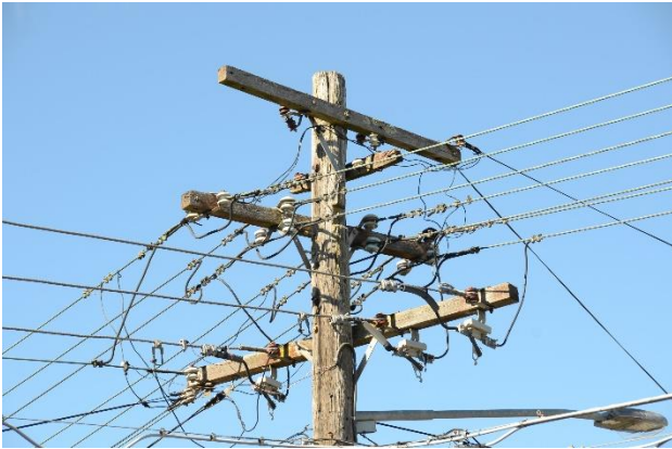
Figure E1: LV under slung links (USL) on pole
