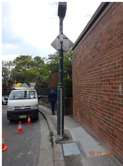
Figure E4: Small Cell antenna installation on metal streetlight standard. Cable installation is external to the pole
