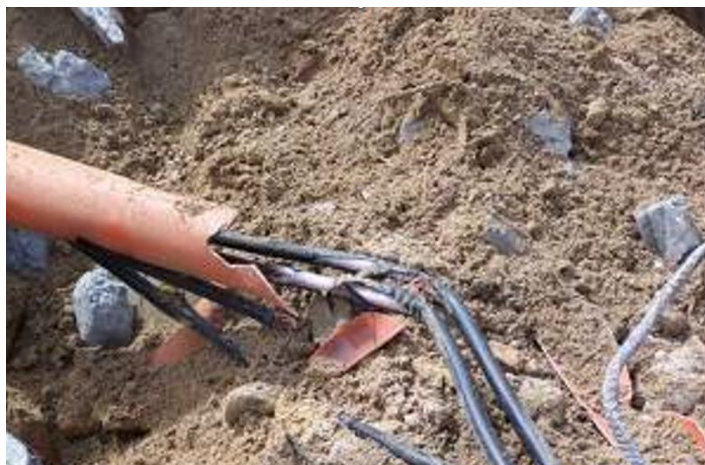
Figure 8: Example of damaged Ausgrid asset
