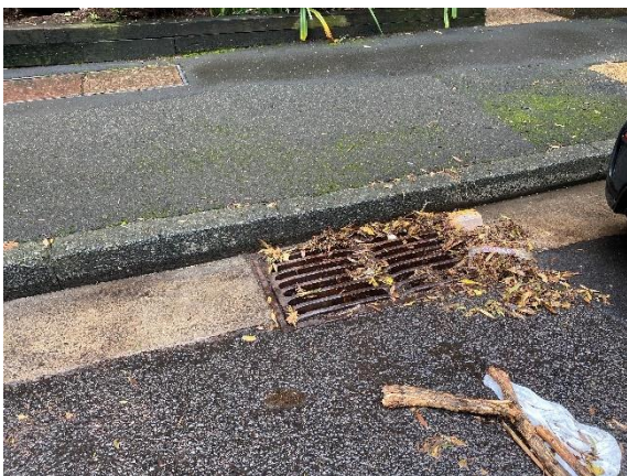
Figure 33. Stormwater drain outside 89 Buckingham Street, in the vicinity of where a stream and sewer were marked on an 1865 plan.
