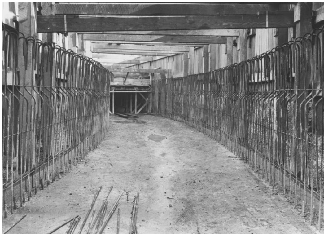
Figure 22. 'View of Stormwater under construction in Waterloo', 1928. A photograph showing the formwork for the construction of the channel underground. Source: Sydney Water Photograph Collection, City of Sydney Archive.
