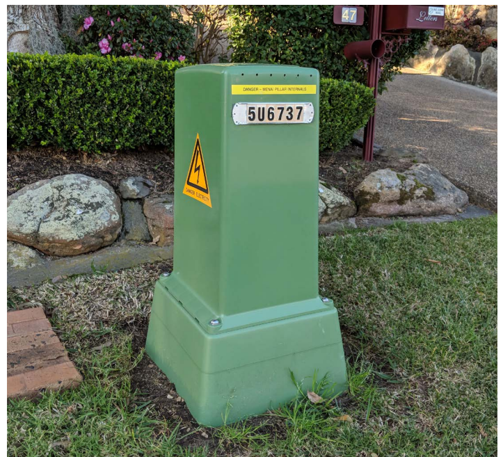
Typical current standard pillar to be installed
