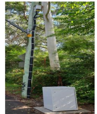
Small Cell Antenna with ground mounted equipment cabinet
