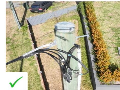
Image of 200Amp Service connected via Bolt and Lug
