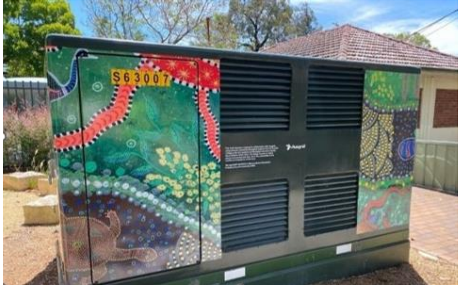
Image of Kiosk substation
