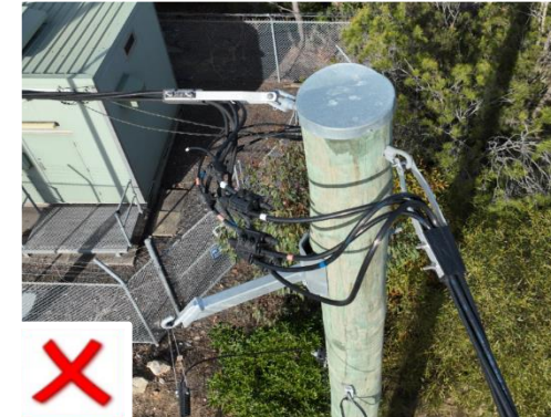
Image of 200Amp Service connected via IPC's
