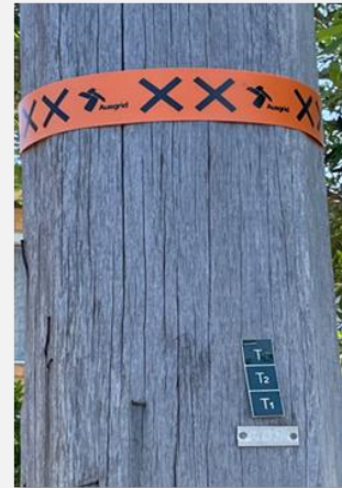
Image of Defective pole marking – Orange Band
