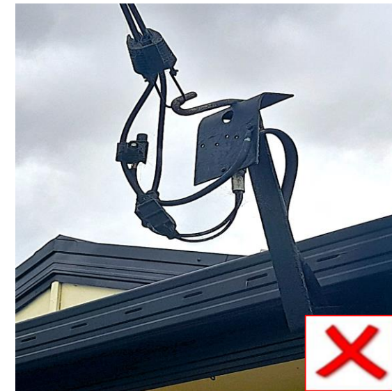
Image of Service Cable Neutral cable bonded to metallic point of attachment bracket
