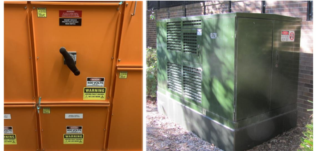
Image of Service protective device and kiosk substation
