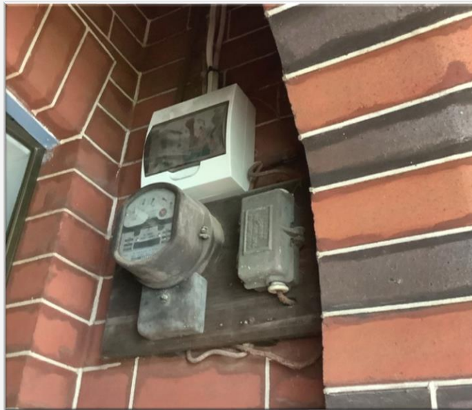
Image of metal clad service fuse
